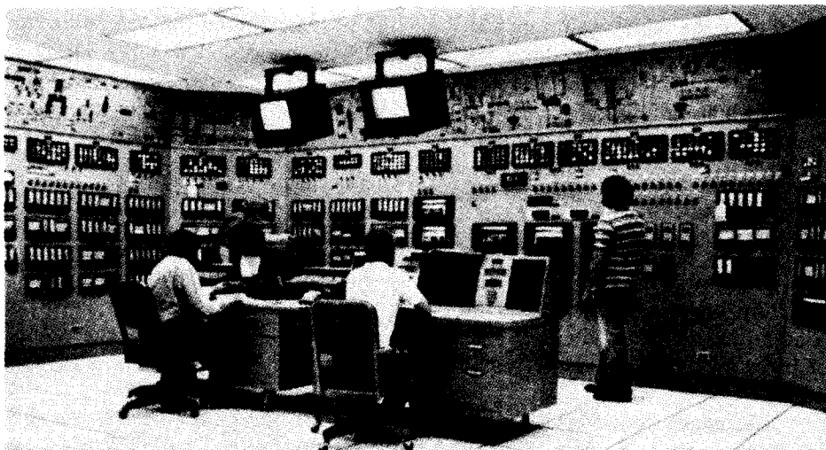
FIGURE 3-4 Example of a graphic panel for a modern industrial plant with a computer-controlled system. (Courtesy of C. F. Braun and Company.)
